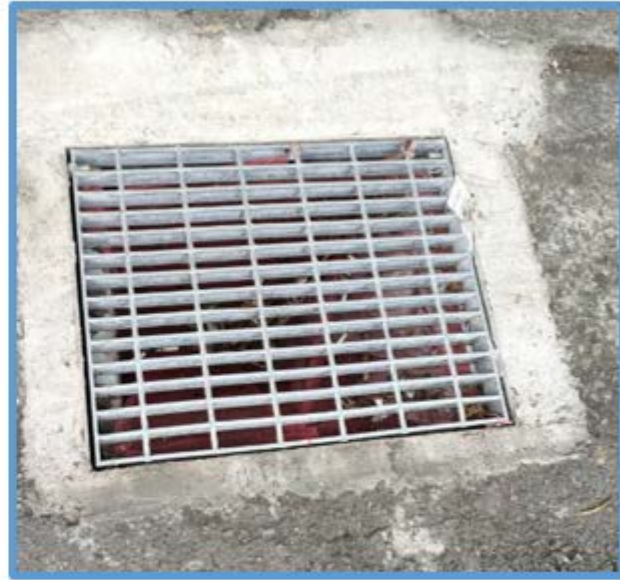
蓋框變形改善情況
